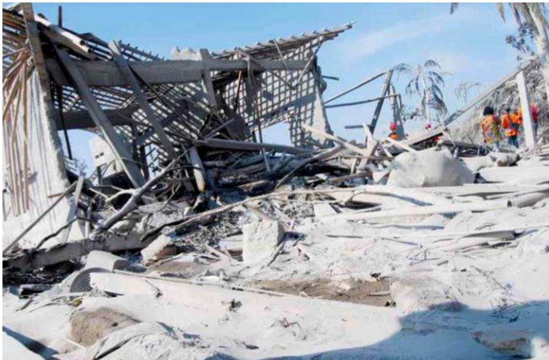
Pict 2. The damage of residence is caused by hot clouds
